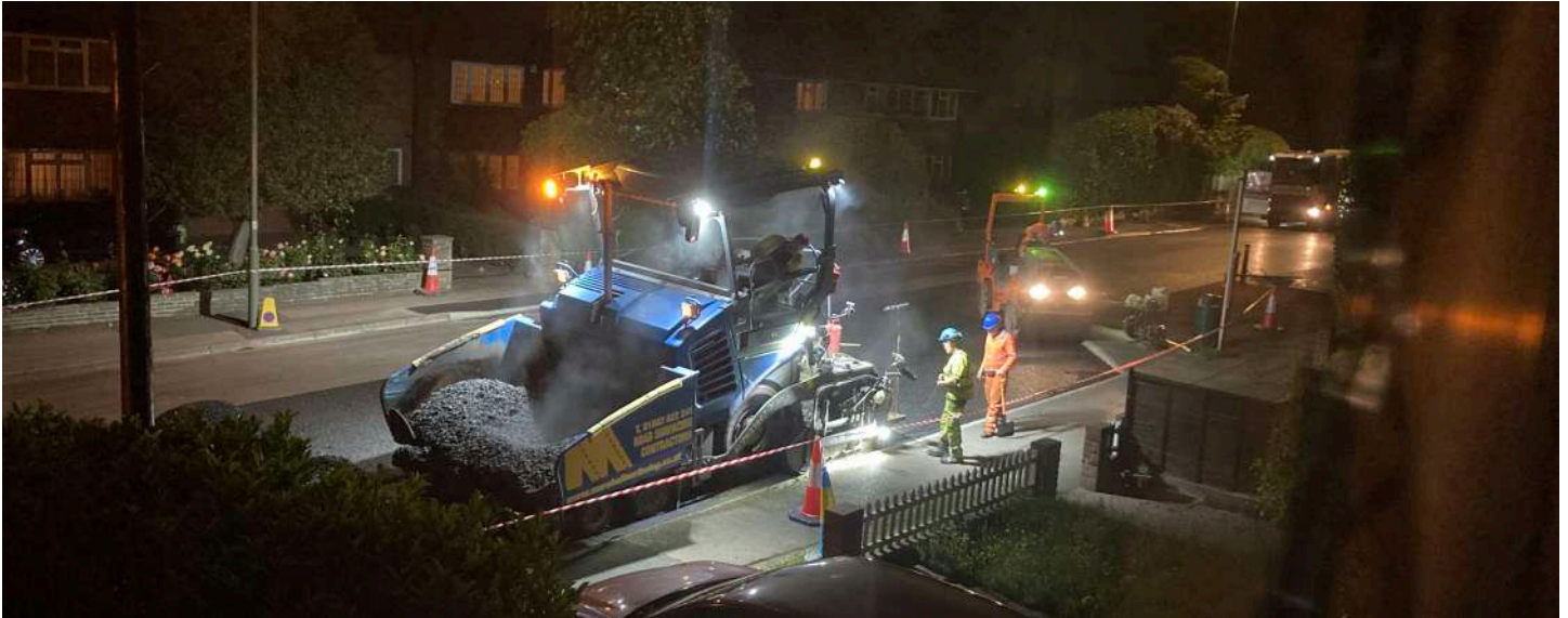
Resurfacing of Hare Lane involved all-night working – minimising disruption, but keeping some residents awake
